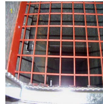
HVAC Supply South Wall 20" x 20"
