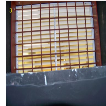
HVAC Return East Wall 12" x 18"
